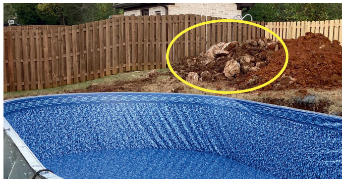
Some jobs have a little rock in the ground when we dig, so be aware that your yard could have the same. It is important for the bottom of the pool base around the outside to have dirt pushed up around it to help contain the sand.
