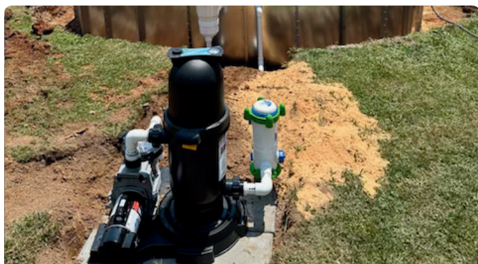
This is a picture of your pump and filter. Notice the dirt ground after digging out the pool. This is very common, and most homeowners plant seed and straw to grow back the grass after installation, or you can use decorative gravel.
