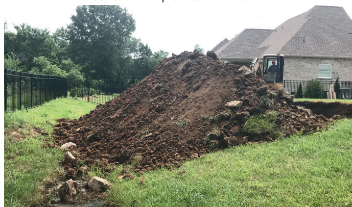
The dirt removed from the hole will be placed in close proximity to the pool so that it will be easier to move by the homeowner once the pool project has been completed.
